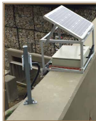
Smart Barrier System 智能泥石壩系統
